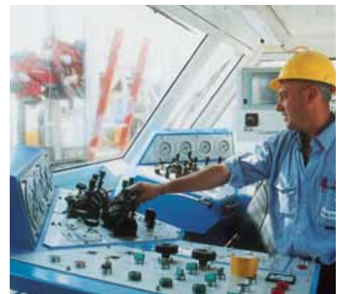
Driller's cabin – Automated drilling console
